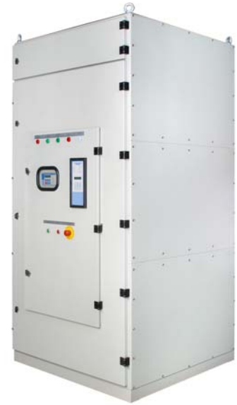
Solcon's HRVS-DN, 6.6KV
