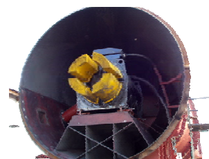
One of the 3m diameter mine exhaust fans
