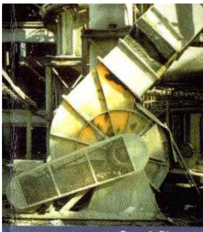
Industrial Blower: 3.3 KV, 80A, 1 MW
